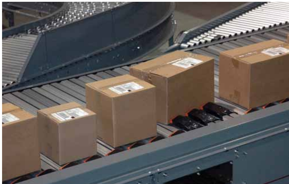
Conveyor and sortation systems are using software and controls to manage the flow of goods while distributing work in a way that eliminates bottlenecks.
